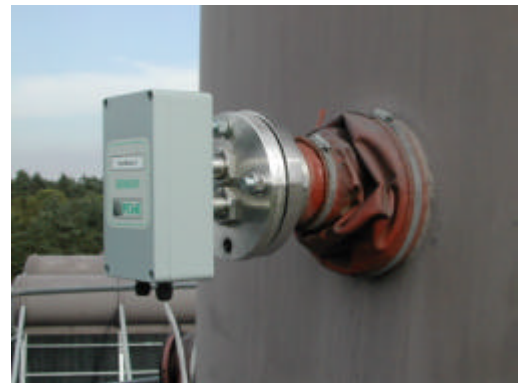
StackMasster II Installation at Power Generation facility
